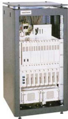
(α) Digital Base Station (DBS)
