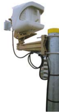
(β) Radio Base Station (RBS)
