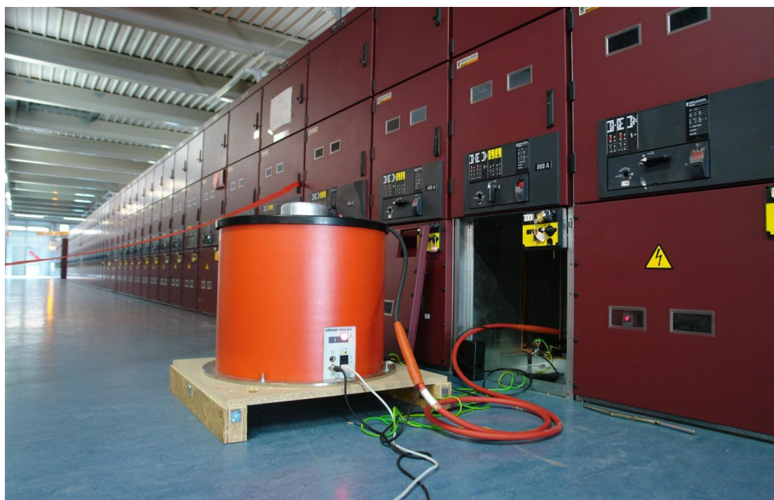
Figure 82: OWTS system while measuring in BE substation the EMD217/BE feeder
