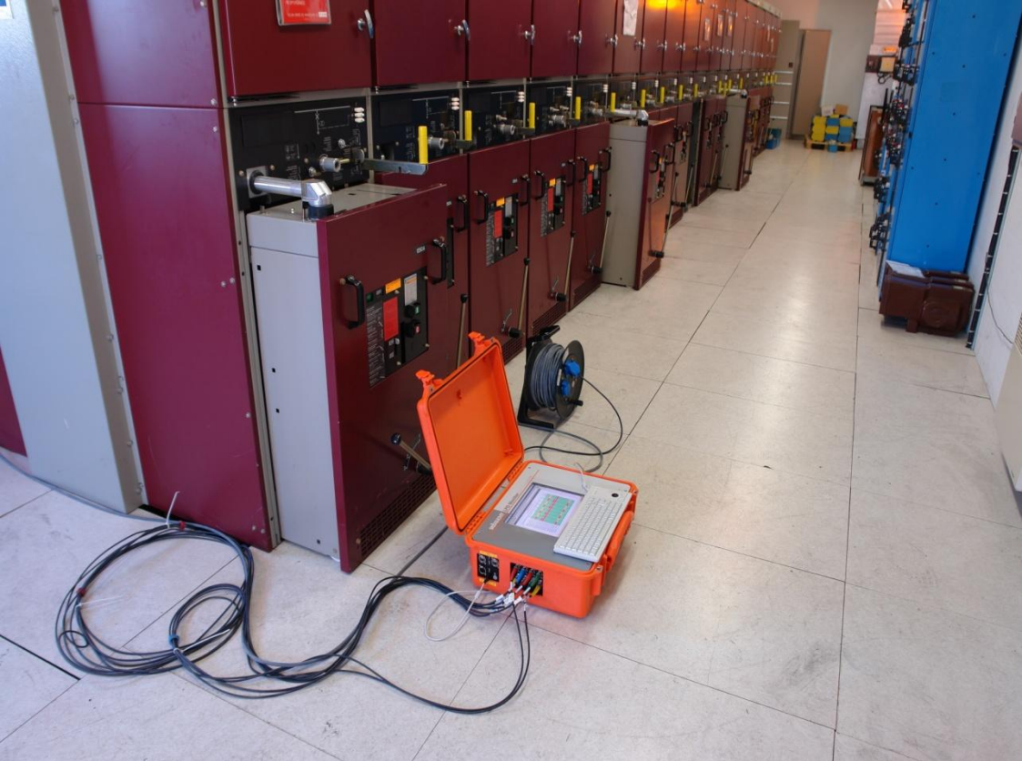
Figure 48: LPD monitor measuring in BE9 substation
