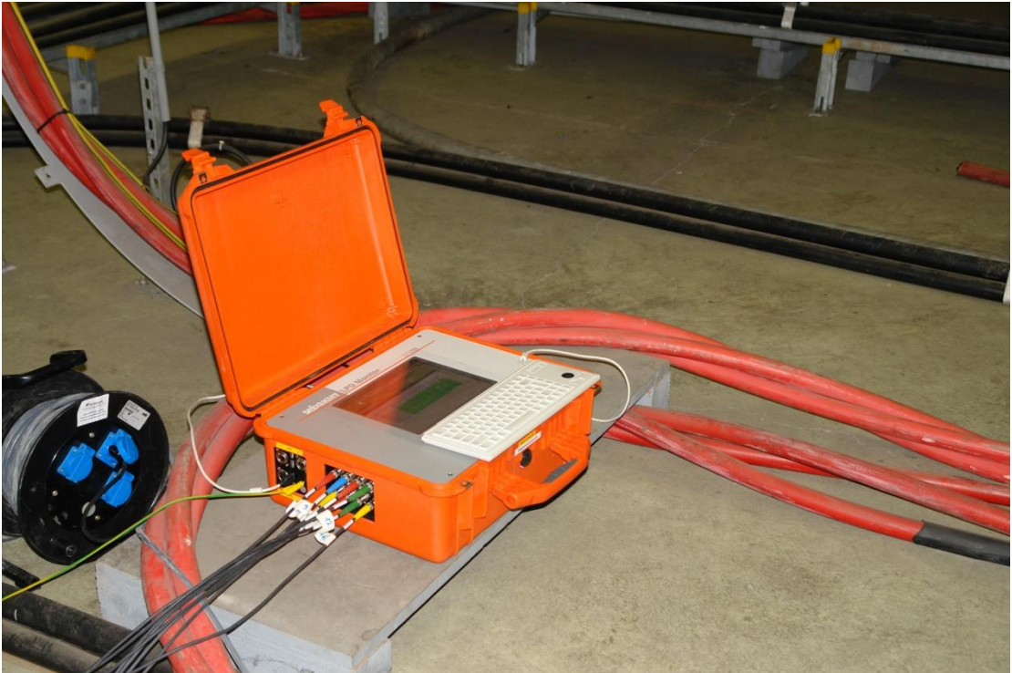
Figure 45: The LPD monitor and the sixteen input sensor cables
