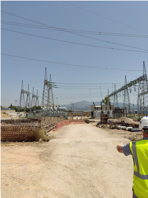
Figure 1.1. Outdoor environment of a high voltage facility in Pallini, Greece.
