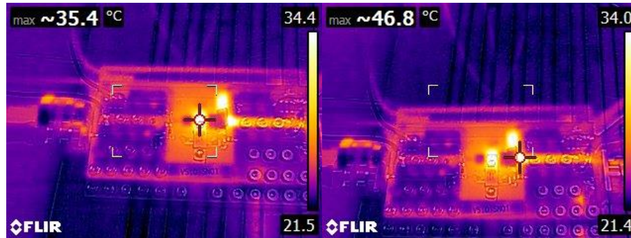
Figure 6.52: Pictures from the thermal camera monitoring the temperature of the transistor and the output coupling capacitor of iteration #5
