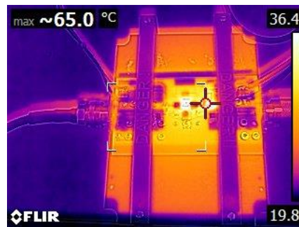
Figure 6.33: Picture from the thermal camera monitoring output capacitor
